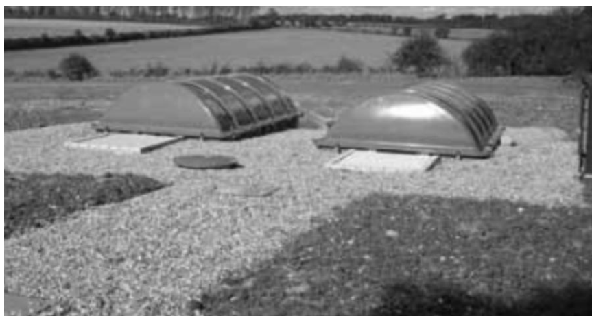
Rys. 3. Oczyszczalnia typu DN16 RBC – Winchester, Anglia Fig. 3. The wastewater treatment plant DN16 RBC – Winchester, United Kingdom
